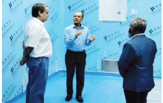
Hon'ble Chairman paying a visit at Annex A construction Site and giving his directives
