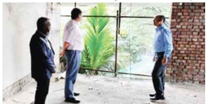
Hon'ble Chairman paying a visit at Annex A construction Site and giving his directive
